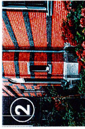
GREY STAIN APPLIED TO BRICK DETAILING ON REMAINDER OF SHOPPING CENTER AND PORTION OF BRICK BELOW STOREFRONT
